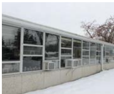
Original windows in need of replacement at Indian Hill
