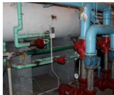
Aged hot water systems and pumps at Maple Dale
