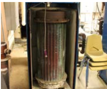
Outdated boiler in need of replacement at Indian Hill
